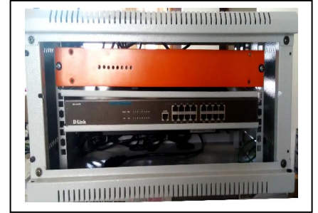
MASTER CONTROL STATION
